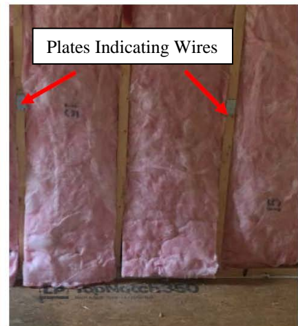
An example of batts not cut to fit wall cavities with plates showing wire locations
