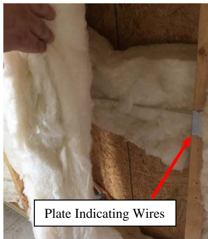
An example of an overfilled cavity with a plate highlighting the wire location
