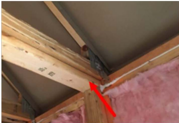
An example of top plate gasket missing on interior walls.
