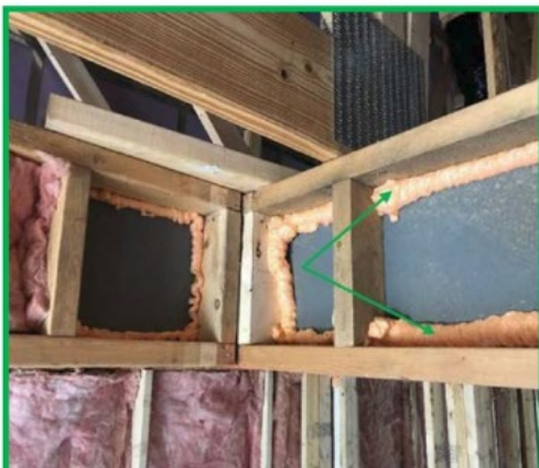
Tray ceiling is fully sealed
